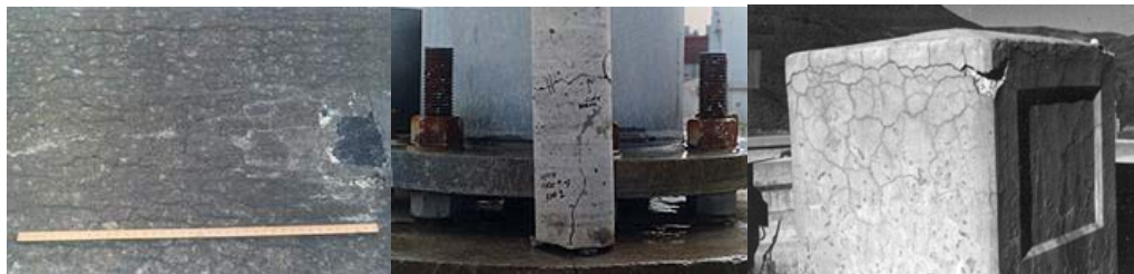
ASR Cracks Formation
